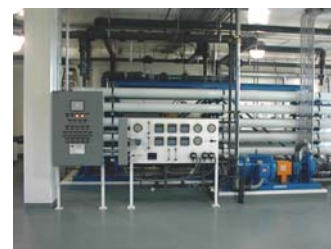
Diversas vistas do equipamento instalado na central. Several views of the equipment installed in the facility.
