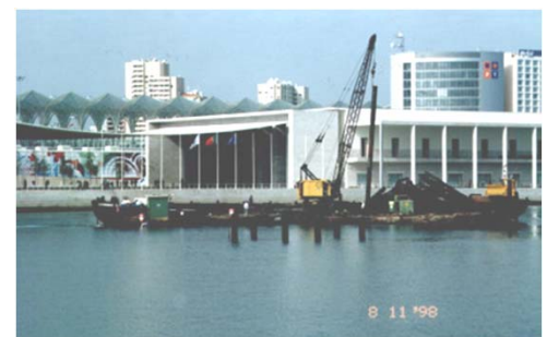
A demolição no fim da festa The party was over: demolition works in progress
