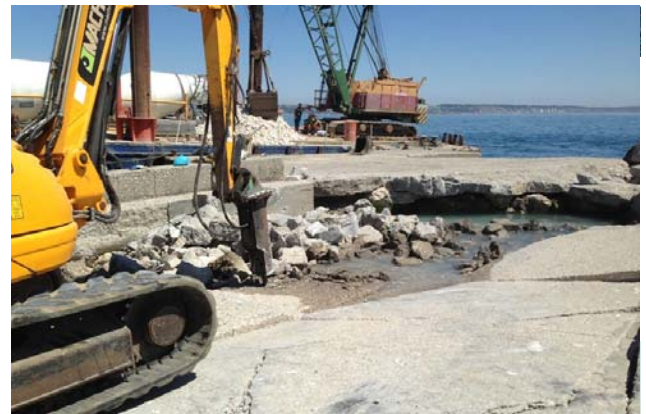
Repair of the void at the Bugio Lighthouse (Photo by Manuel Garcia)
