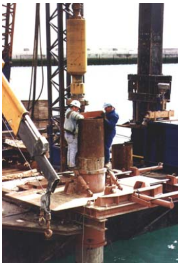
Special foundations: marine pile driving (tubular and sheet). SETH is the undisputed leader of this sector in Portugal
