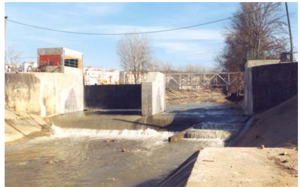
Inflatable at Arrabalde: view downstream of the two spans, cofferdam and house to electrical controls
