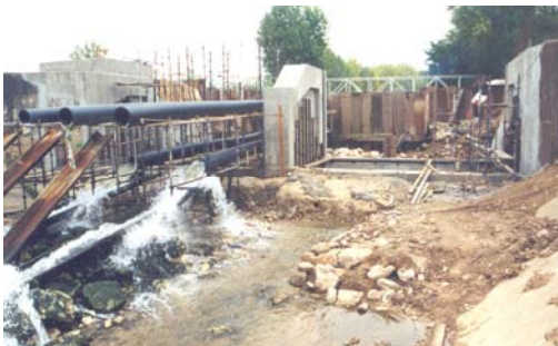
Inflatable weir at Arrabalde: river to flow only in the lower tubes, during the execution of work
