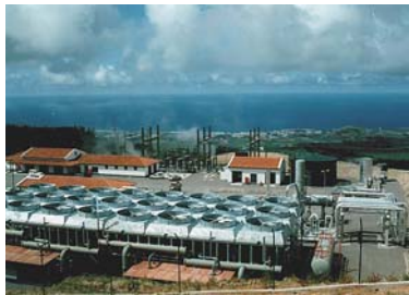
EDA - Geothermal Plant at Ribeira Grande S. Miguel - Azores
