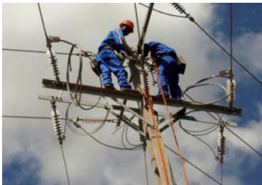
Electricity III, Inhambane Mozambique
