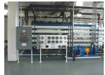
Diversas vistas do equipamento instalado na central. Several views of the equipment installed in the facility.
